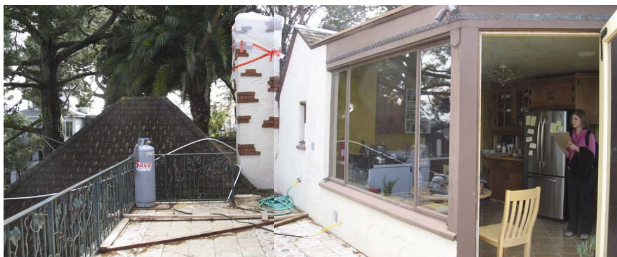
Figure 7. East façade of second story, looking south from northeast corner of deck. Hip roof of southeast addition is visible at left. (Source: Page & Turnbull)
